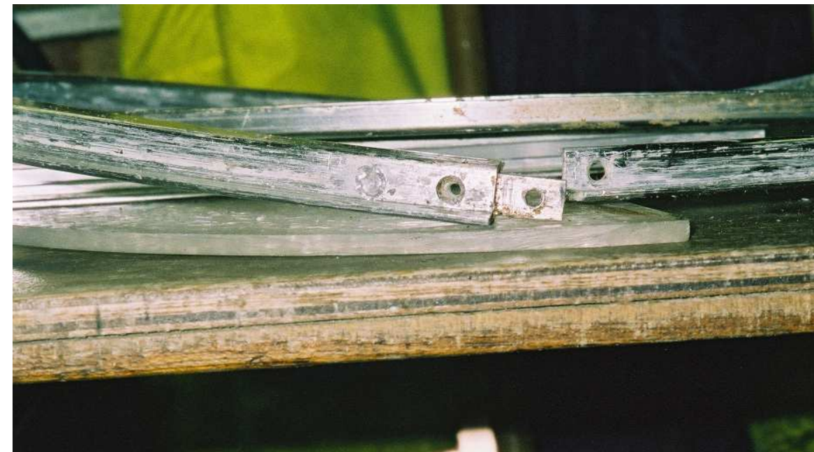
This picture shows where the frame comes apart and the old screws removed.
